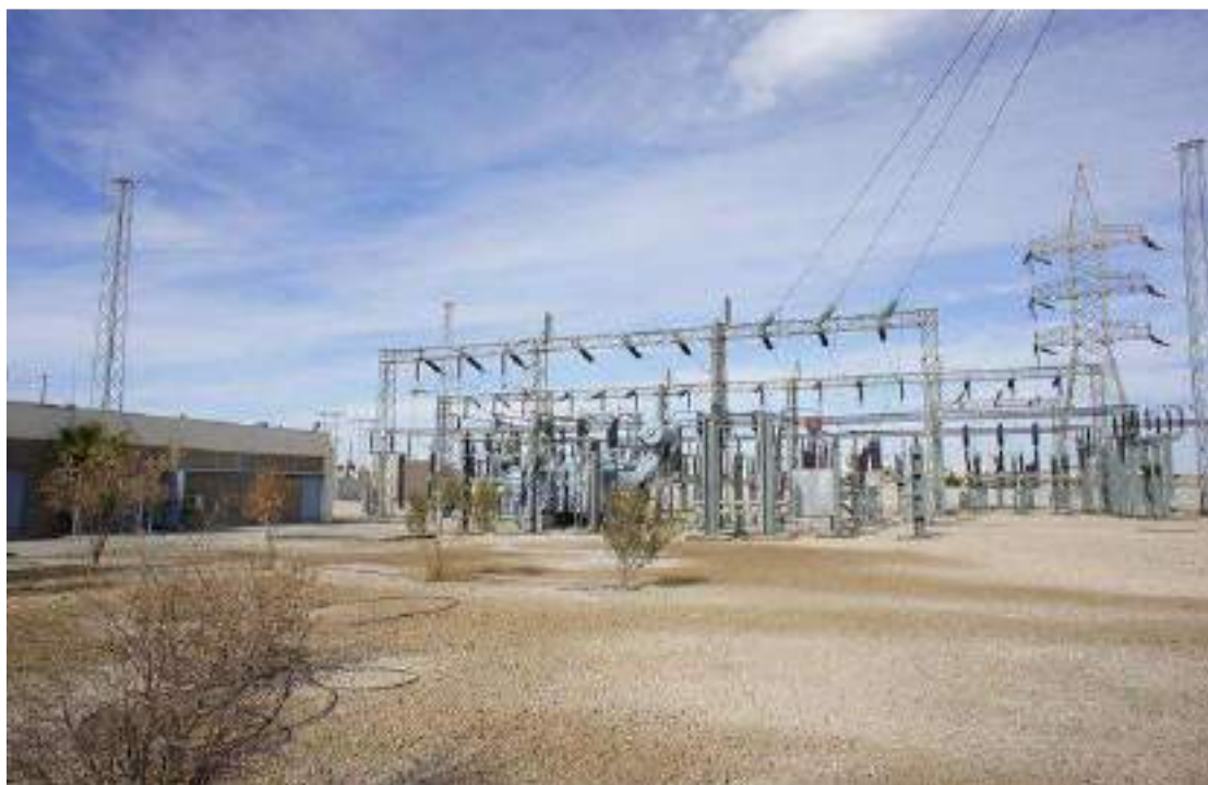
Figure 11: Typical 33/132kV Substation
