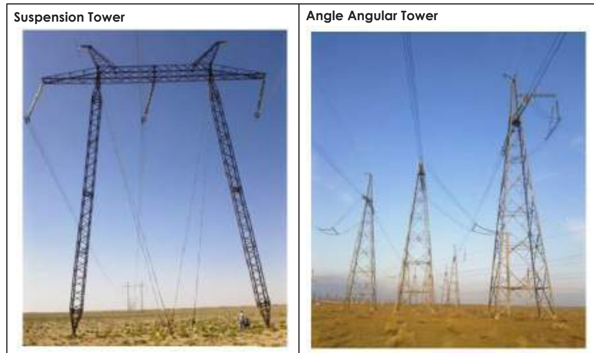
Plate 2-26 Example of Typical 500kV Suspension & Angle Angular Towers
