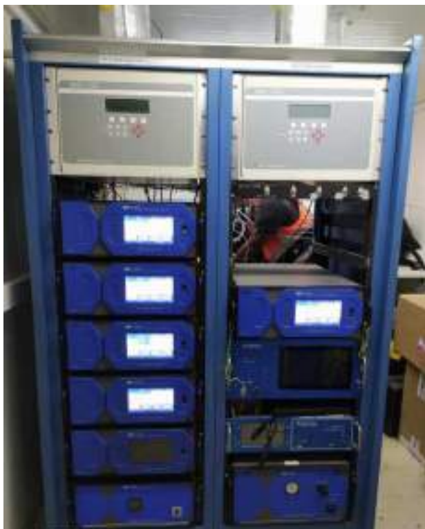
Fig. 3. Overview of the rack of instruments at AQ mobile
