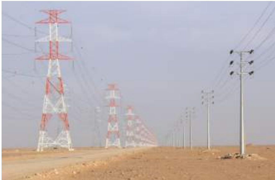
Figure 4-5: Overhead Power Lines
