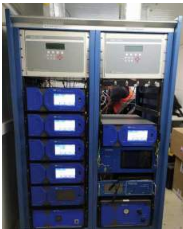
Figure 4.61. Rack in the Air Quality mobile station
