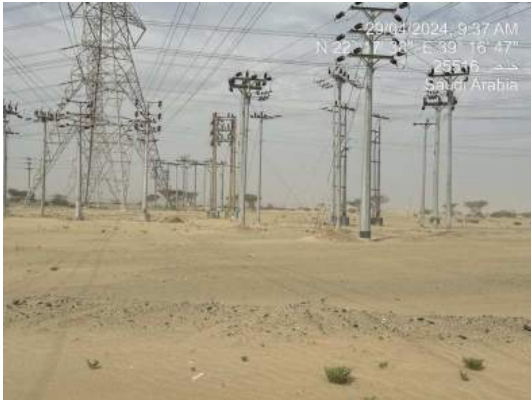
Figure 4.54. Photograph of the electric line in the project site.
